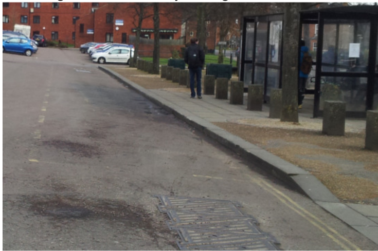
Fig3 Camber at the bus stop – which results in bus doors coming into contact with the ground sometimes jamming the door mechanism.
